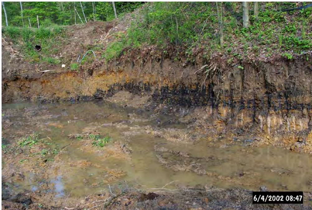
A portion of the Oxyc Limestone Drain during excavation. Note the coal seam along the bank.
