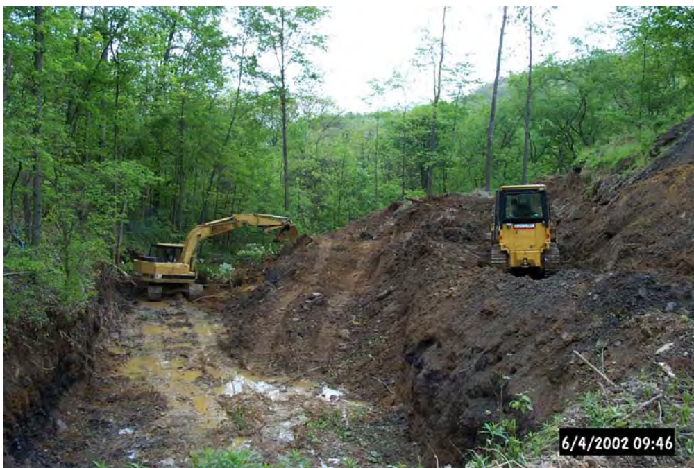
Jesteadt Excavating removing a portion of the spoil in order to construct the diversion channel around the Oxic Limestone Drain.
