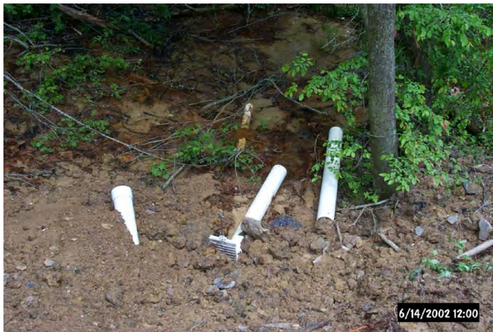
The outlet pipe from the Oxidic Limestone drain, which will discharge into the wetland is located on the left while the flush valve and flush pipe is located in the center.
