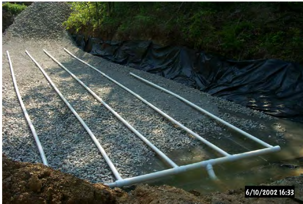
The underdrain flushing system for the Oxidic Limestone Drain.
