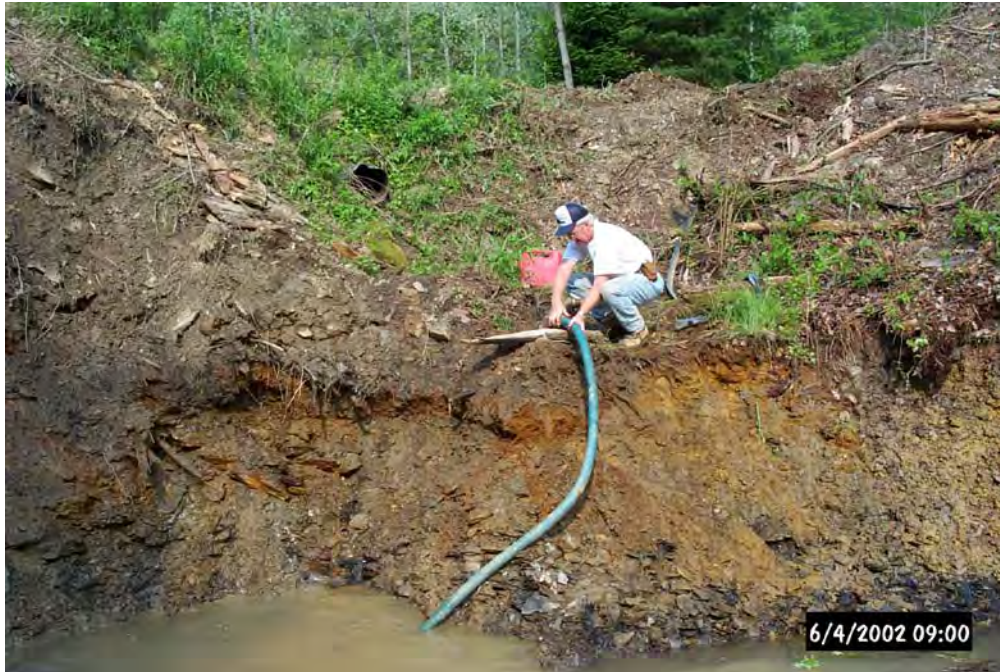
Jerry Jesteadt, owner of Jesteadt Excavating, pumping out water that has collected within the sump for the Oxic Limestone Drain.
