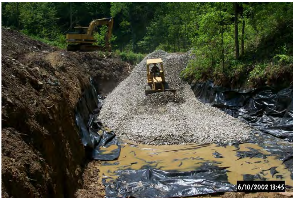
Placement of the AASHTO #1 90% \text{CaCO}_3 limestone in the Oxidic Limestone Drain by Jesteadt Excavating.
