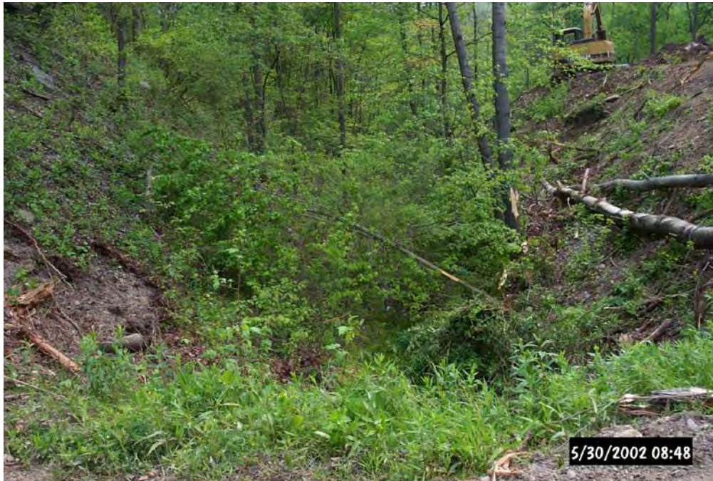
View of the vegetated spoil breach and source of the abandoned mine discharge during site preparation for the construction of the Oxyc Limestone Drain passive treatment system.
