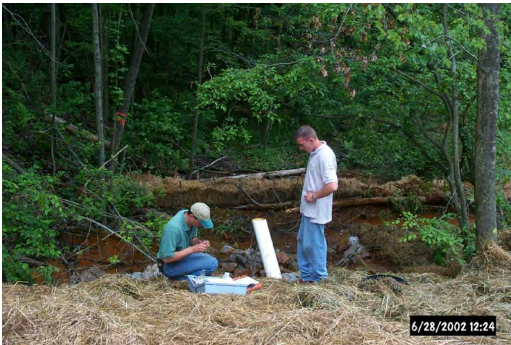
Tim Danehy and intern Steve Short, Stream Restoration Incorporated OSM intern, checking the alkalinity of the effluent of the Oxidic Limestone Drain.
