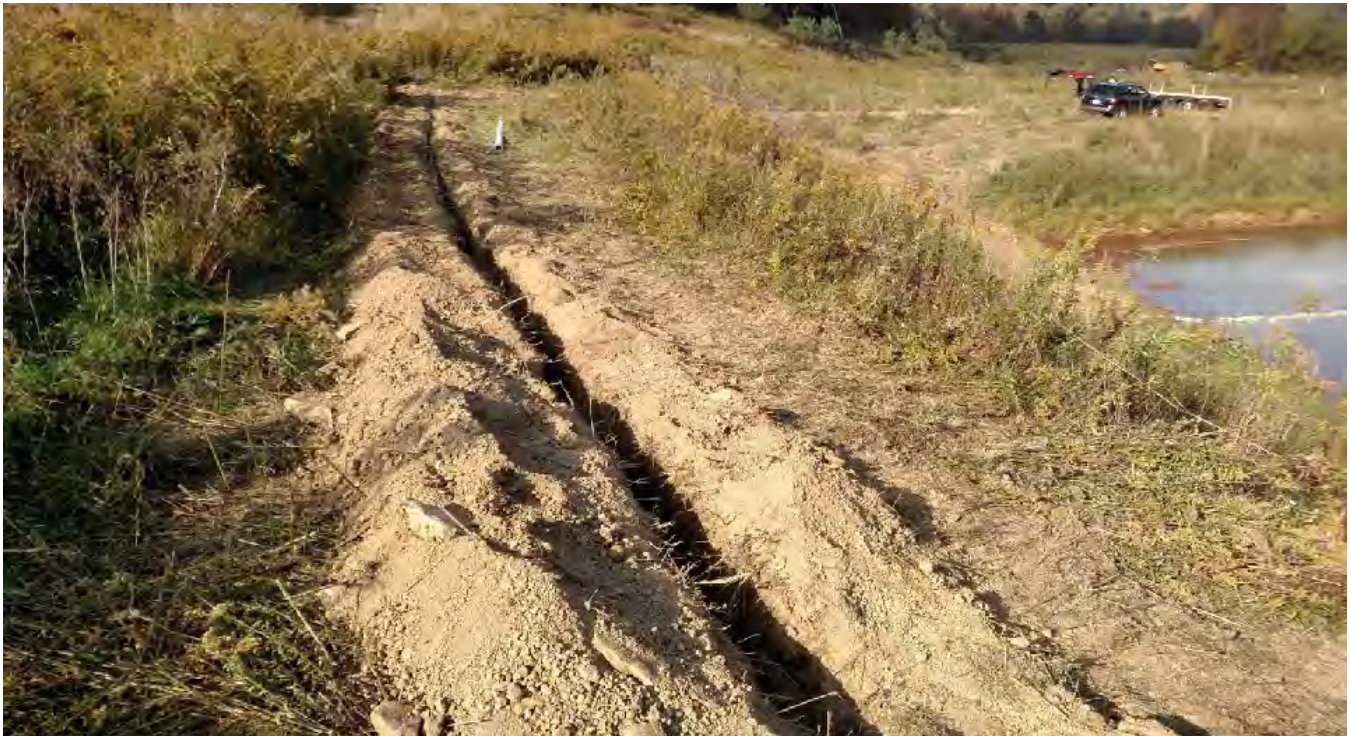
Top: Airline above pond #3 looking downhill as airline extends from shed area. Bottom: Airline above ponds #2 & #3.
