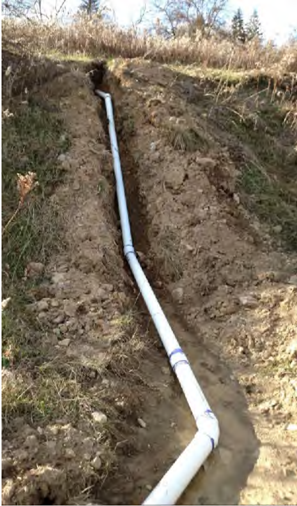
Left: Looking uphill at airline from valve box at pond 1. Bottom: Looking downhill at airline towards manifold box at pond 1.
