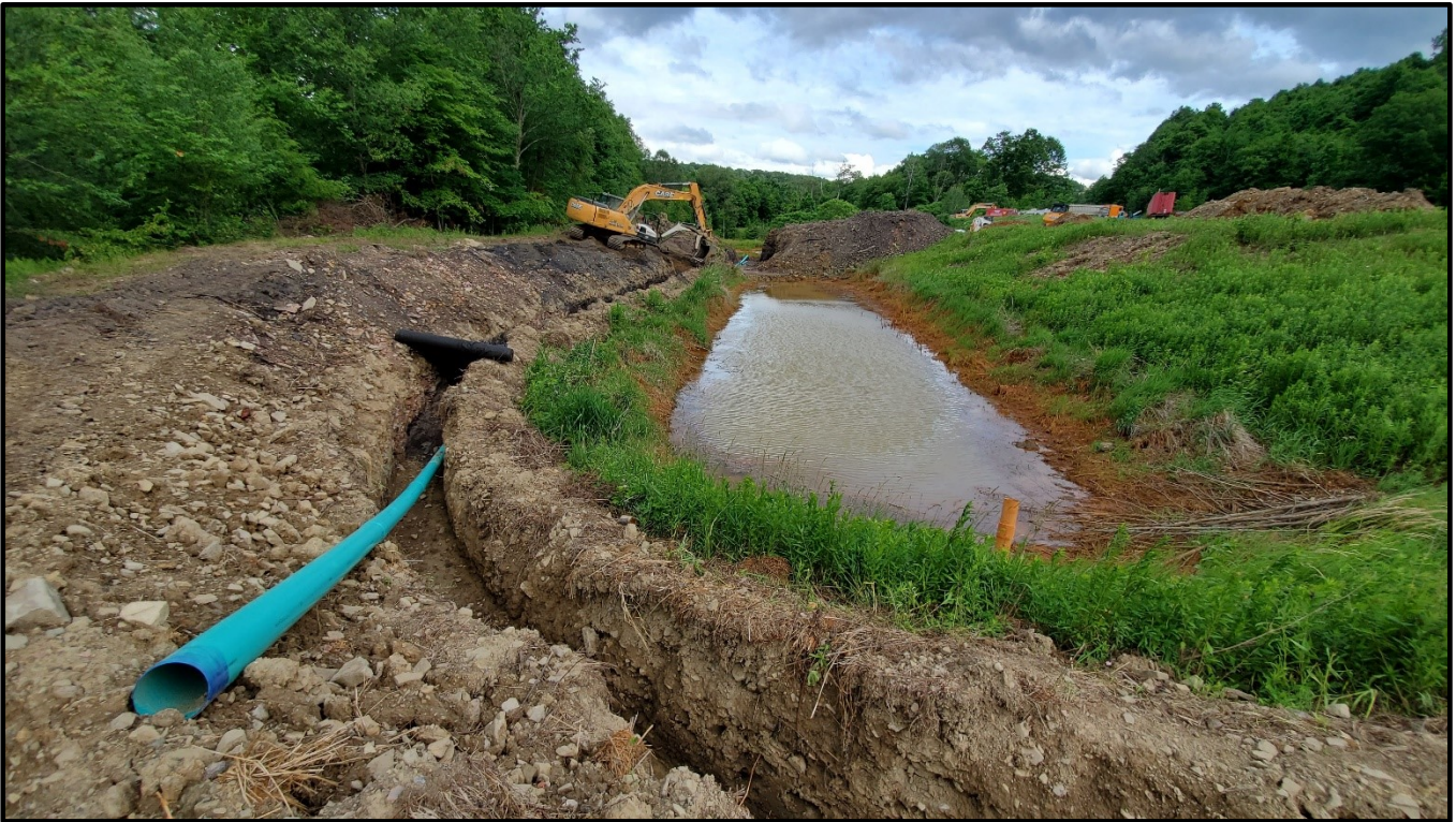
Top: French drain pipeline (solid portion) extends along the north slope of JVFP3 and outlets to the Wetland (6/18/20).
