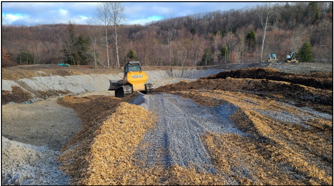
Top: JVFP1 with exposed underdrain outlets pipes before pipe was installed through the berm, filter stone was installed and leveled except for the area near the exit, and stockpiled media can be seen in the background (12/04/20).
