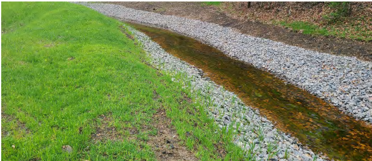
Top Left: Terraced iron formation (TIF), also known as oxidation precipitation channel (OPC), installed at the inlet Ferris West treatment system that treats the SR85/86 discharges. (2022)
