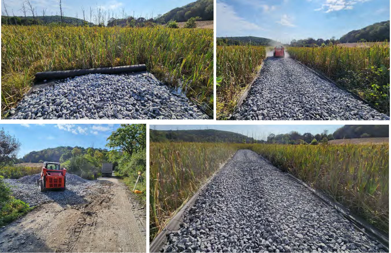
Top Photos: Construction of the rock distribution berm in the natural wetland which receives flow from the SR81 passive system. (2023)
