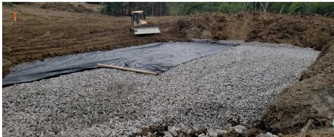
Top Photos: ALD D was excavated by Spur Excavation, LLC to evaluate the quantity of remaining limestone. (2023)
