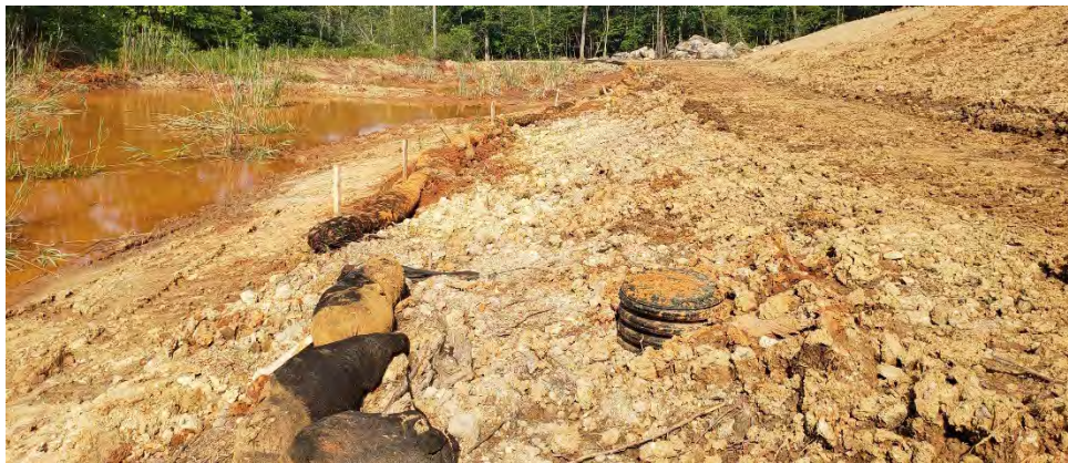
Top: Due to the soft soil conditions and deep sludge, specialty equipment such as the track truck pictured was used to transport sludge and debris from Pond D1 (right) and Wetlands D2 to D4 (left) to the dewatering basin. (2023)
