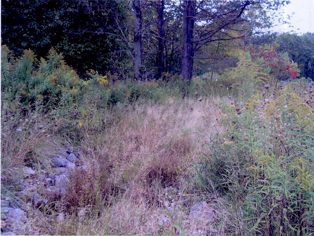
Rock lined ditch (looking down slope) directing flow to the SAPS pond. Note the amount of overgrown brush on ditch invert and side slopes. Date of Photo: 10-2-08.
