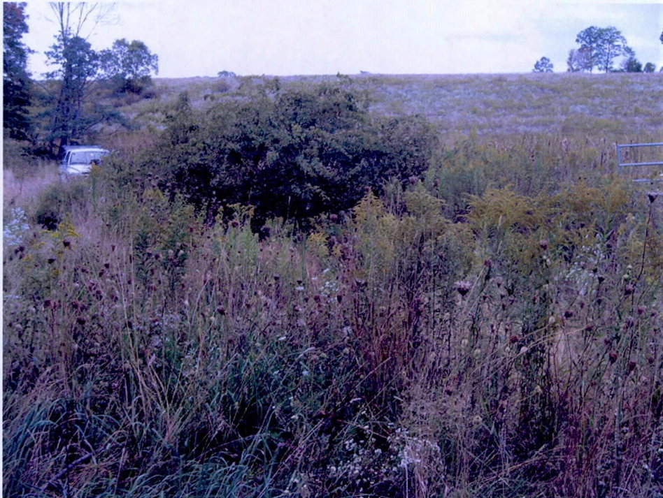
Rock lined ditch (looking up slope) directing flow to the SAPS pond. Rock lining not visible due to overgrown brush. Date of Photo: 10-2-08.
