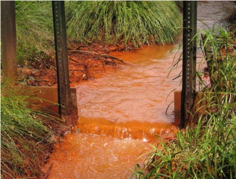
Photo D. The Markle weir. The absence of a stilling area makes measurements using standard weir charts inaccurate.
