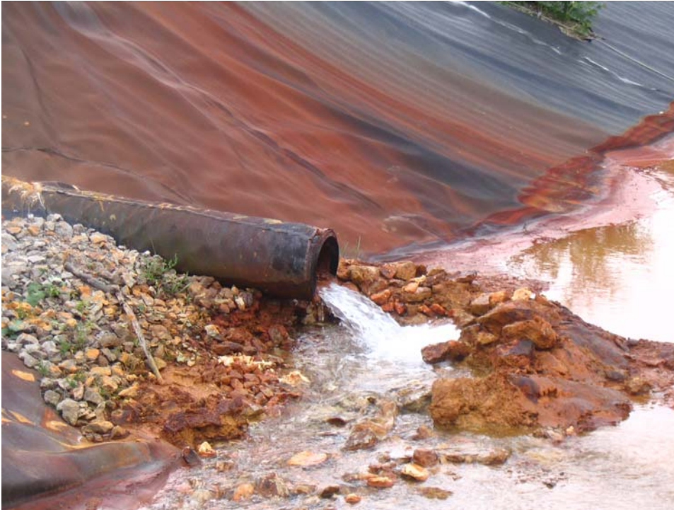
Photo E. The ALD discharge to the settling pond. Note the pool made in the aggregate to accommodate a flow measurements with a 16 gallon tub.
