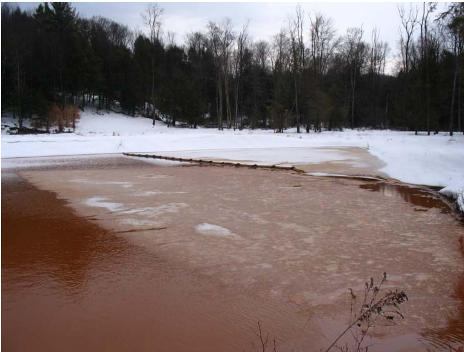
Photo B. View from the emergency spillway to the south. The effluent pipe (located at the end of the pond) was plugged, making this portion of the pond ineffective (as indicated by the ice buildup).
