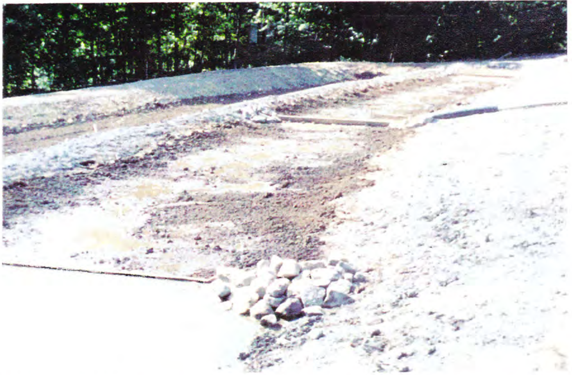
BEFORE PLANT ESTABLISHMENT A mixture of Composted Biosolids and Pond Cleanings (silt) are saturated with treated acid mine drainage shortly after the collection channel wetland was seeded with a mixture of 24 different wetland plant species. Jennings Environmental Education Center, Butler Co., PA (8/97)
