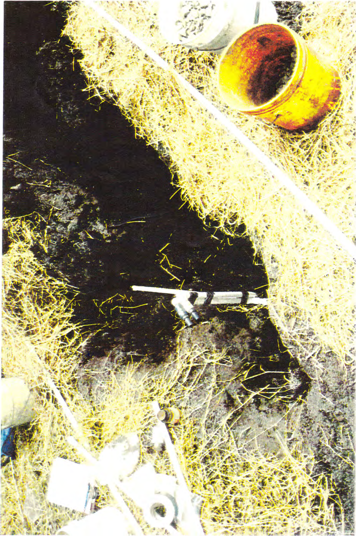
SAMPLING PORT INSTALLATION Two sets of sampling ports placed at varying depths within the treatment media of the full-scale vertical flow system at Jennings Environmental Education Center. Samples can be obtained to investigate the changes in water quality as it passes through the ~2' of treatment media. (c. 7/97)
