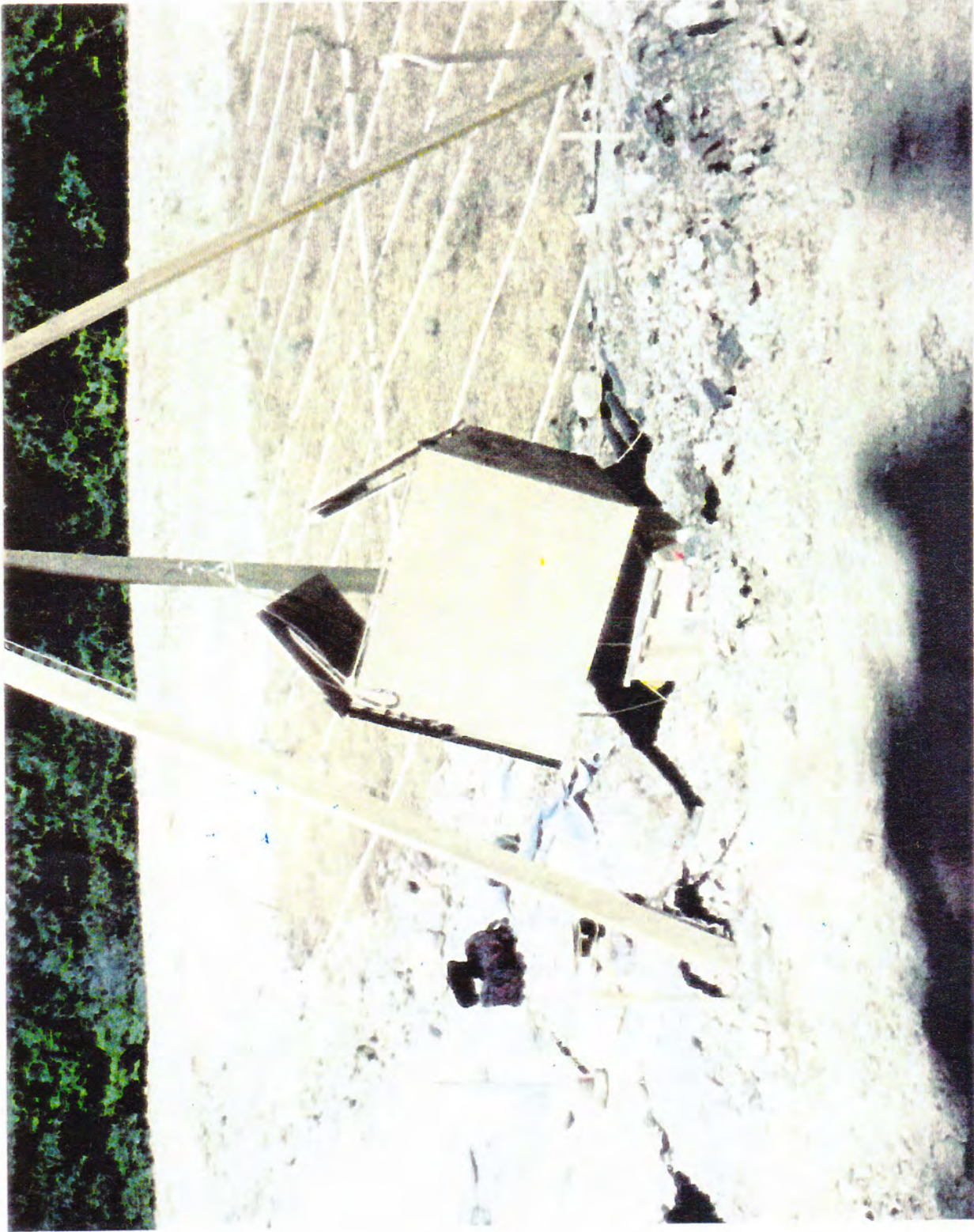
MANUAL PLACEMENT OF FLOW SPLITTER BOX MANHOLE used to house a specially designed flow control device which delivers the flow to an overdrain system evenly distributing the aluminum and iron-laden discharge over the spent mushroom compost and limestone treatment media. (c. 8/97)
