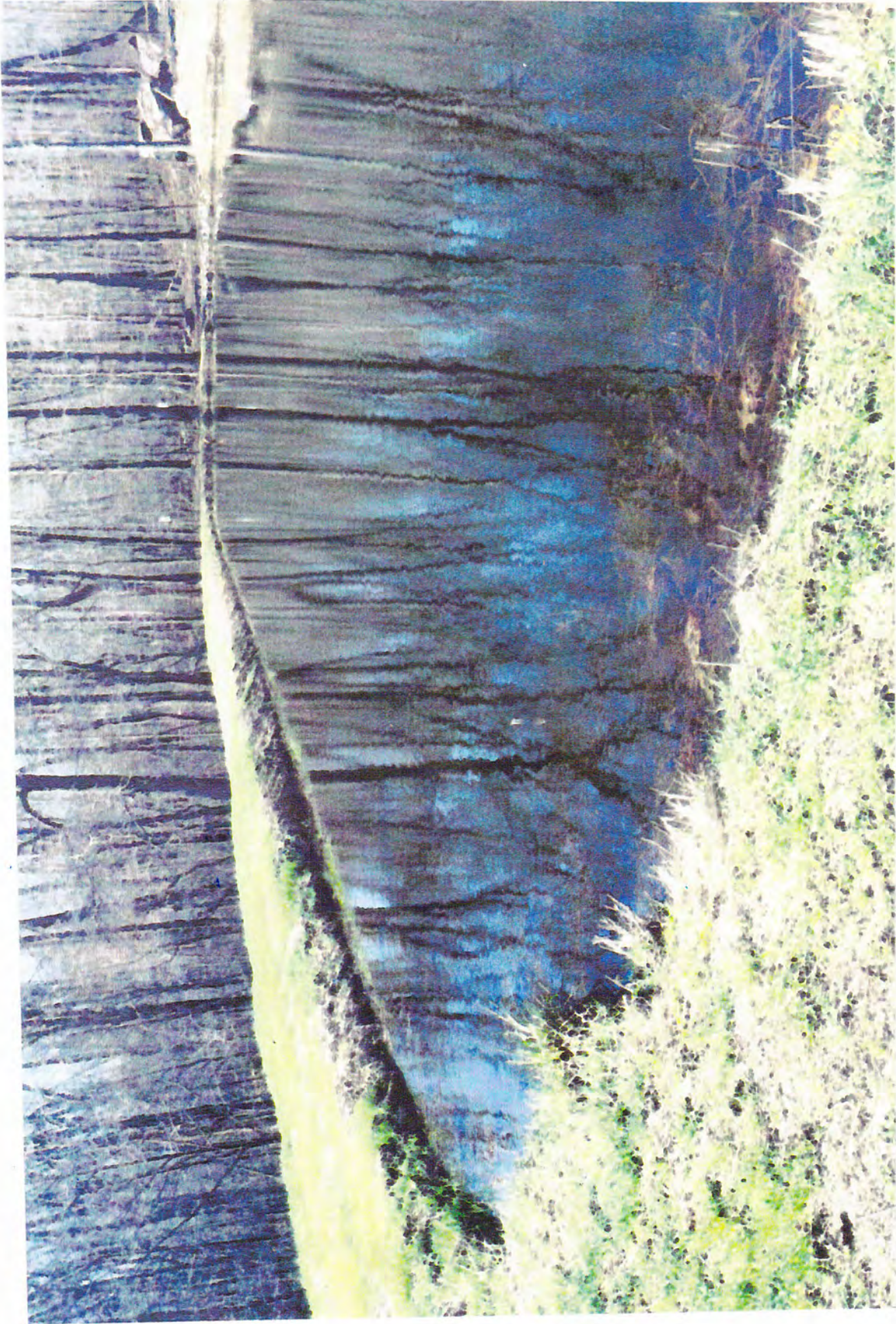
FULL SCALE VERTICAL FLOW SYSTEM AT JENNINGS ENVIRONMENTAL EDUCATION CENTER (PA DCNR). A mixture of spent mushroom compost and limestone is used to treat an aluminum and iron-laden discharge. (4/14/99)
