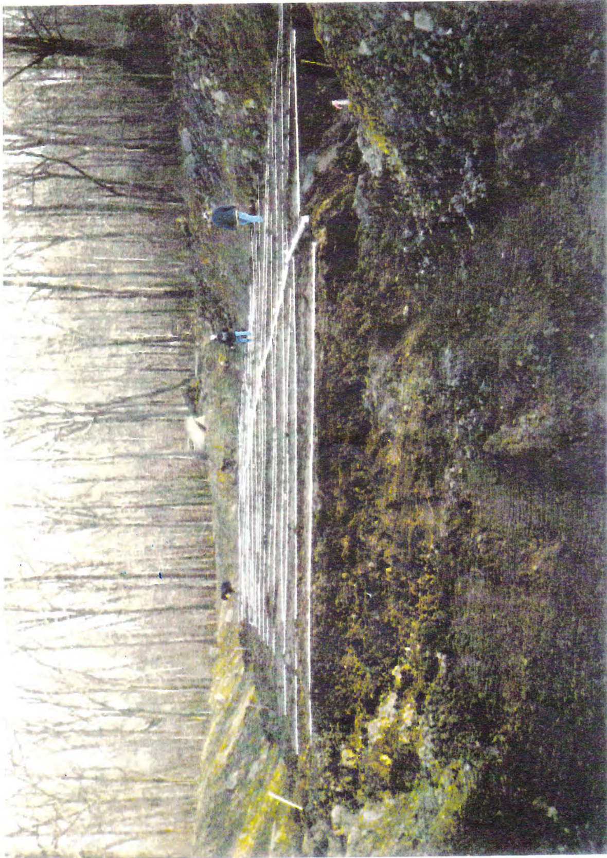
CROSS SECTIONAL VIEW of the full-scale vertical flow system at Jennings Environmental Education Center. Slippery Rock University students are finalizing the installation of the overdrain by leveling the 3/4" laterals which are used to evenly distribute the discharge over the entire area of the spent mushroom compost and limestone treatment media. (c. 5/97)
