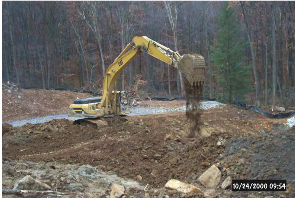
Construction of the B1B3 flush pond that will retain the metal solids during flushing events of the B1B3 Vertical Flow Pond.
