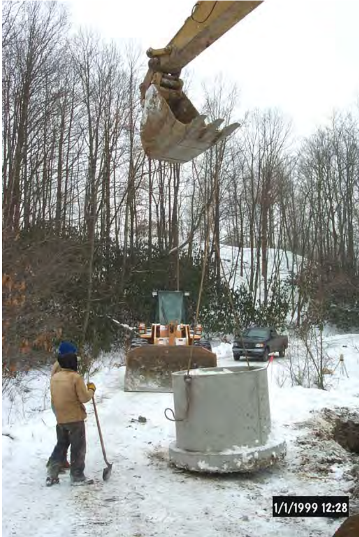
Installation of the diversion well by Amerikohl Mining Inc. at the Harbison Walker Phase II site.
