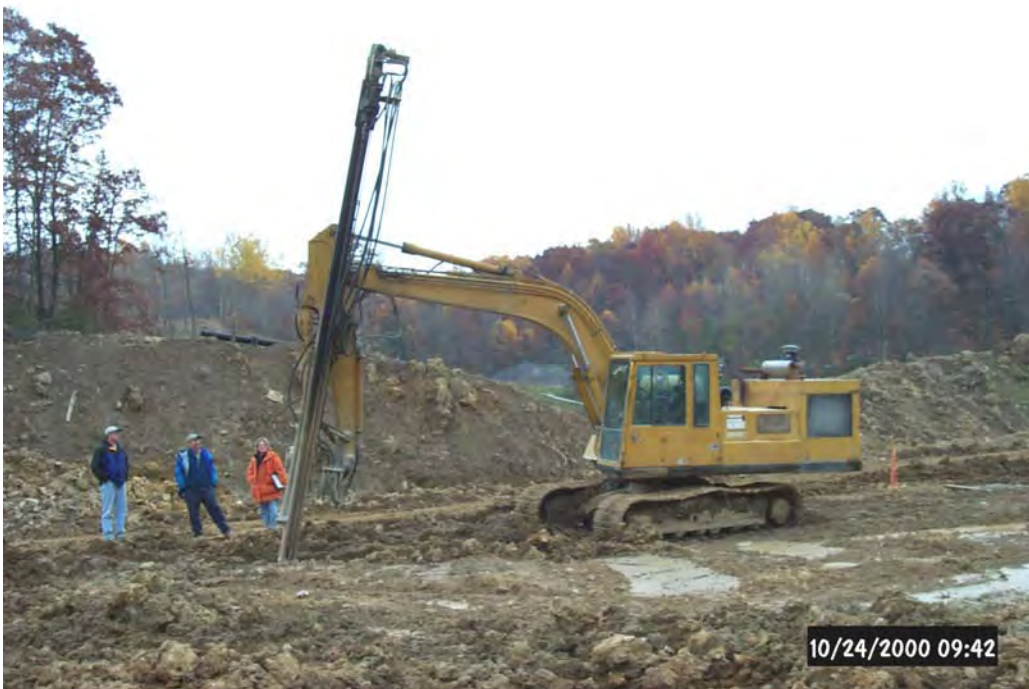
Drilling and blasting were necessary in order to construct the passive treatment system.
