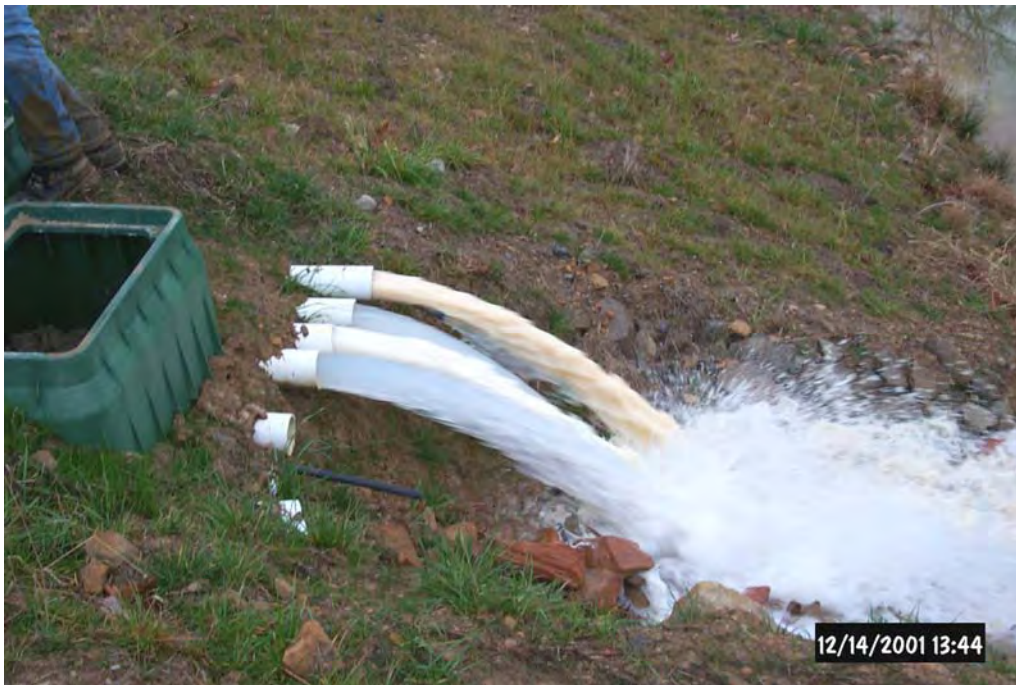
Flushing of the A/C Vertical Flow Pond. Note the white-colored aluminum-bearing, water.
