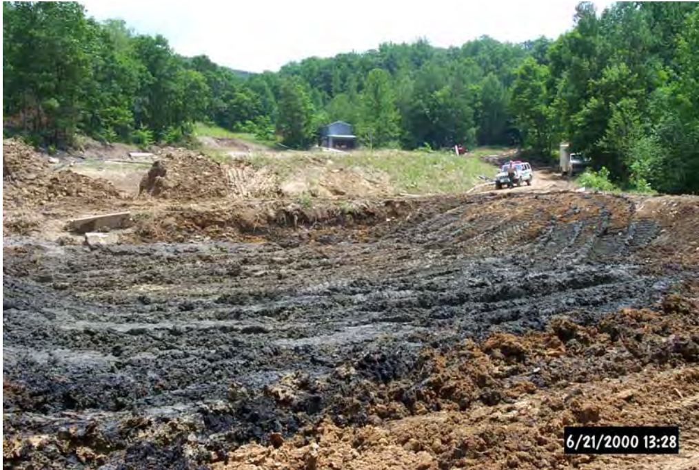
Before the Harbison Walker Phase II Passive System could be constructed, the active treatment ponds had to be pumped out.
