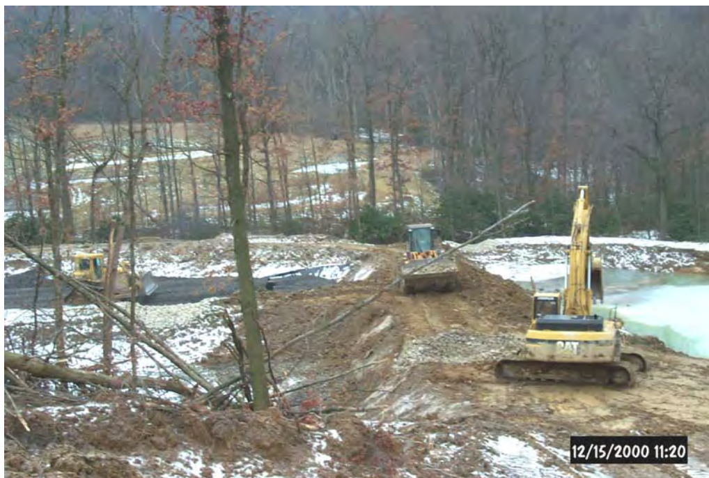
Construction of the A/C system including placing of limestone in the Vertical Flow Ponds left and in the spillways right.
