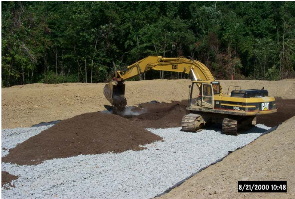
Placement of spent mushroom compost on top of the limestone for the De Sale Phase II Vertical Flow Ponds.
