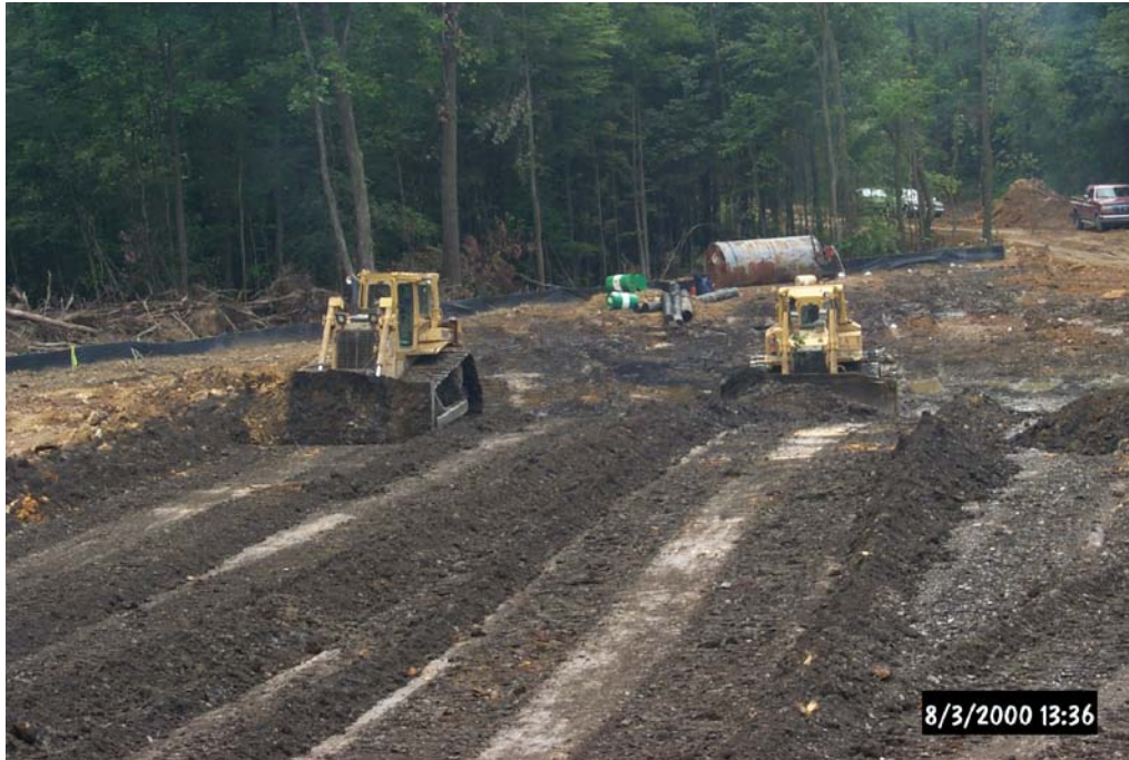
Construction of the Vertical Flow Ponds located in parallel at the De Sale Phase II Restoration Area.
