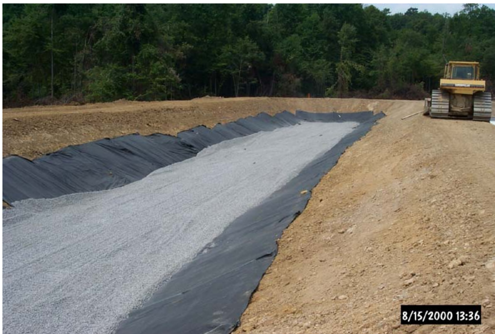
Construction of Vertical Flow Pond West of the De Sale Phase II passive treatment system. Note the geotextile liner and placed limestone.
