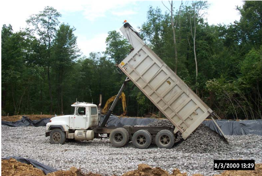
Placement of stone during the construction of the Horizontal Flow Limestone Bed at the De Sale Phase II Passive Treatment System.
