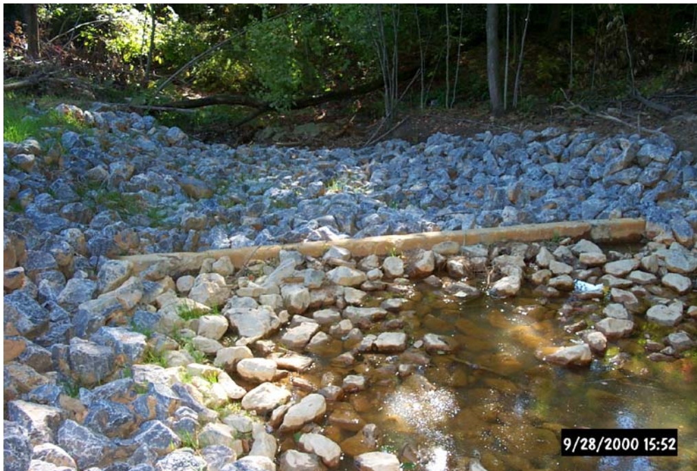
View of the approximate 3-foot high dam (above) constructed of concrete Jersey barriers in order to back up the stream to allow the intake pipe (below) to convey up to 200 gpm of the unnamed tributary into the passive system for treatment. Under normal flow conditions the entire stream is being treated by the passive system.
