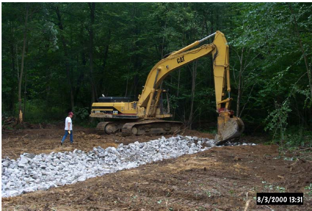
Construction of the final spillway, which conveys the effluent from the Horizontal Flow Limestone Bed to the unnamed tributary of Seaton Creek.
