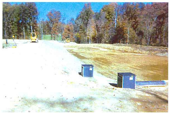
Pond/wetland construction. Inline water level control structures for the Limestone Pond are visible in the foreground.
