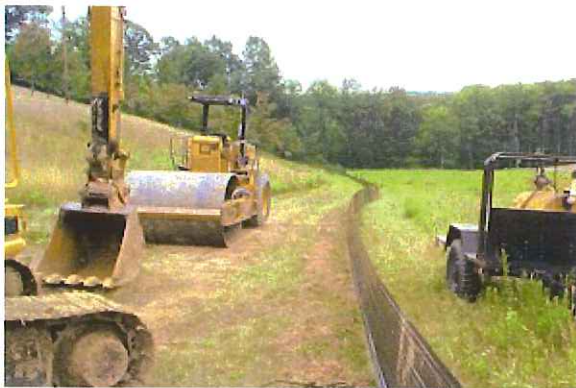
Pipe route to treatment system.
