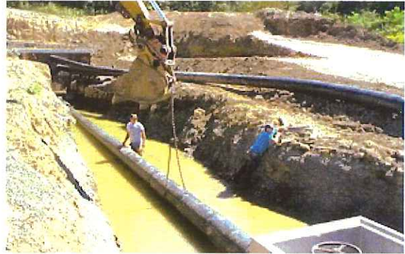
Installing pipe between storm water control structure (upper left) and valve box (lower right).
