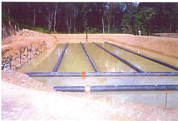
View of flushing network in Limestone Pond prior to limestone placement. Note bedrock exposed on left pond berm.
