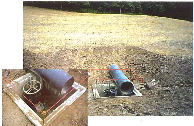
Overview of emergency overflow pipe and valve box (inset) after back filling.
